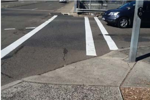
Ryde Road (at Burns Bay Road) not aligned
