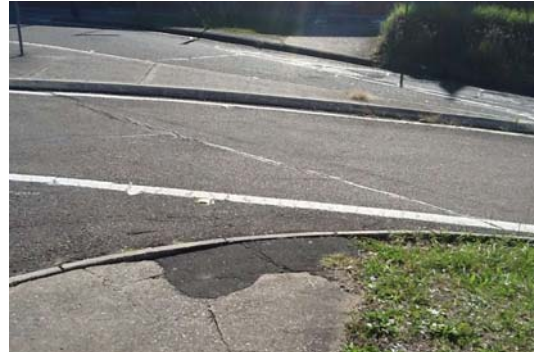
Ryde Road (at Burns Bay Road) missing kerb ramps
