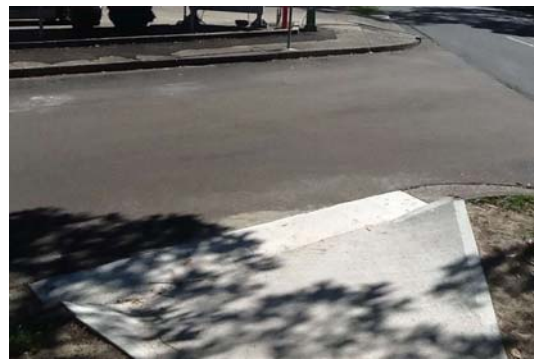
Ryde Road (at Matthew Street) missing kerb ramp
