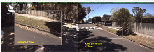
Earl Street, Hunter's Hill: Kerb Distortion
