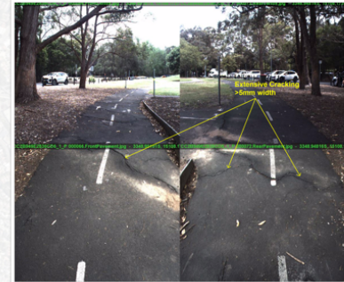
Buffalo Creek Reserve, Hunter's Hill: Footpath Cracking
