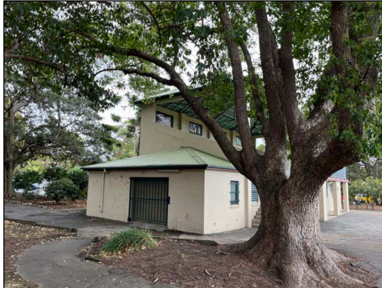
Figure 12 Boronia Park Pavilion – eastern elevation storage room as viewed from adjacent to Park Entry
