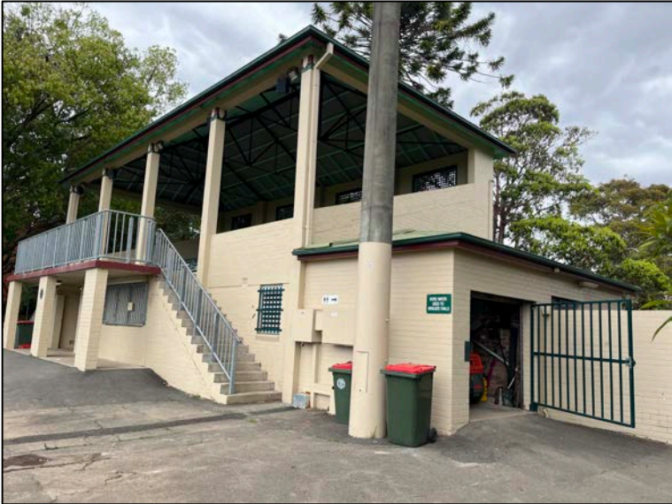
Figure 11 Boronia Park Pavilion – western elevation storage room as viewed from the Park Cricket Oval
