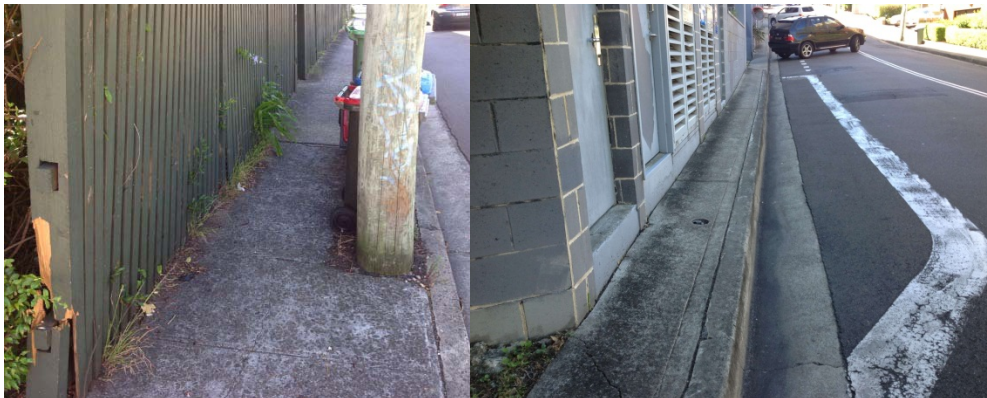
Photograph 32 Existing Footpath Deficiencies, Flagstaff Street
